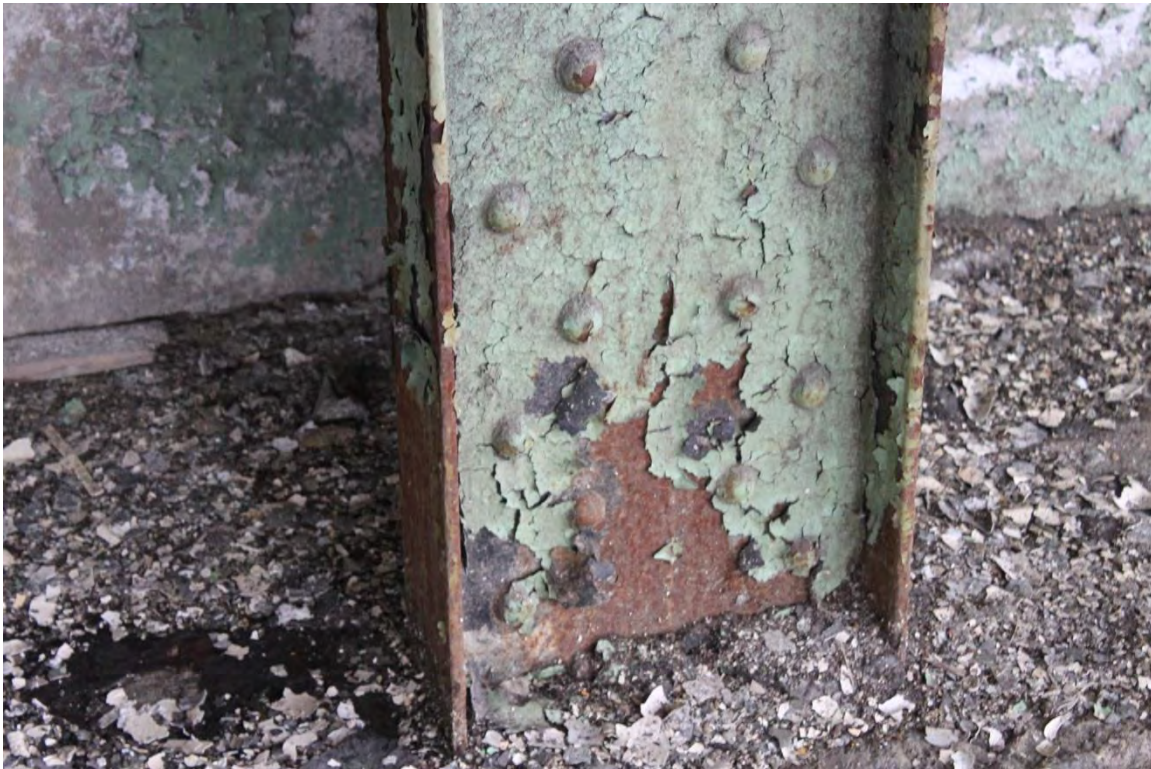
Figure A-15 View of deterioration at base of columns
