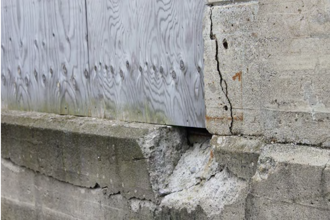
Figure A-14 View of deterioration and cracking
