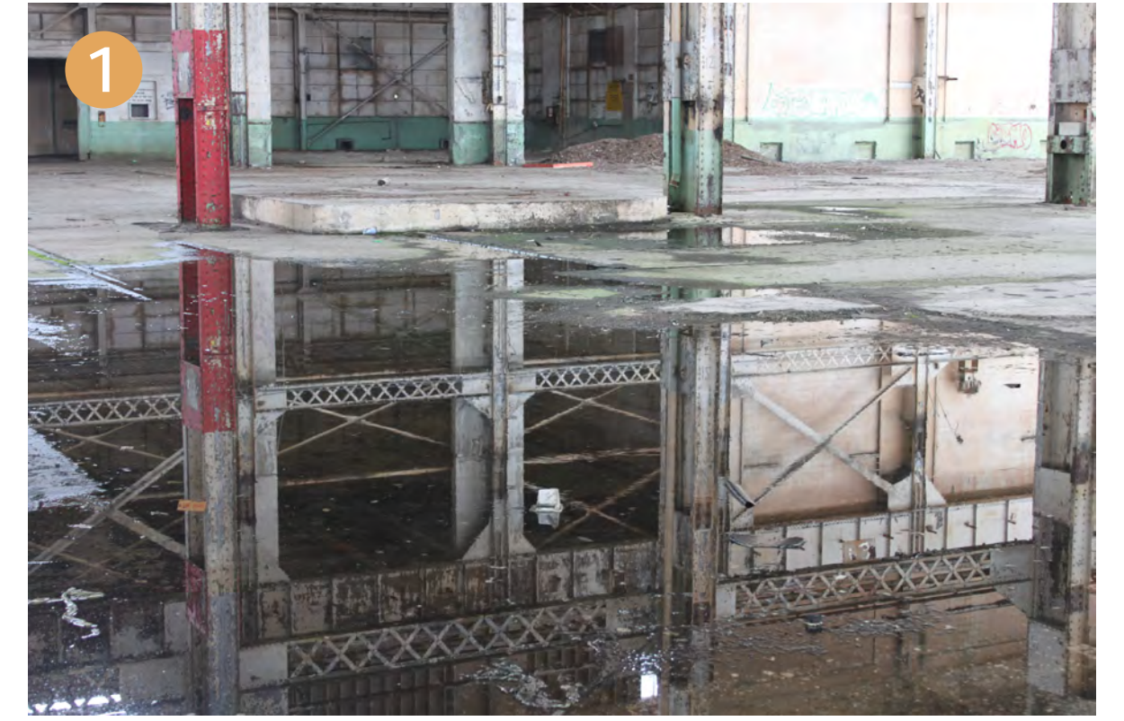
Lack of roofing and large roof openings have allowed water to leak through.
