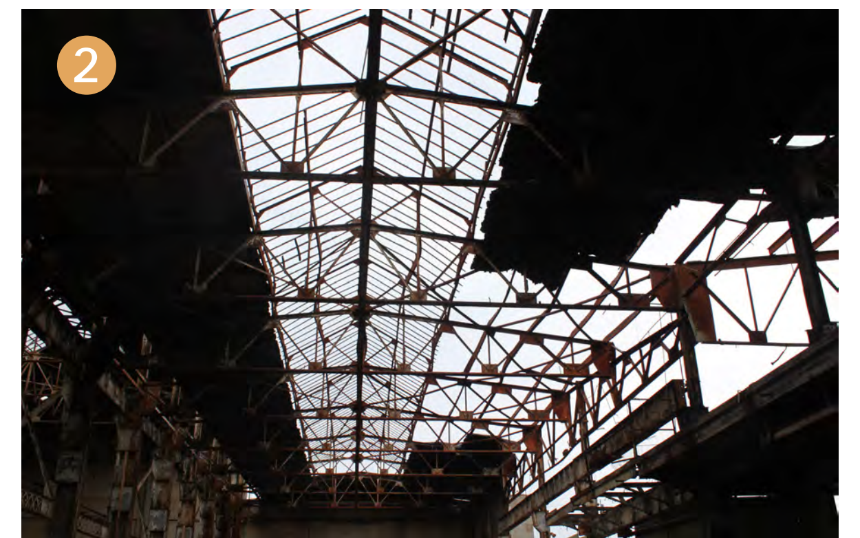
Cladding and roofing systems were found to be in poor to very poor condition.
