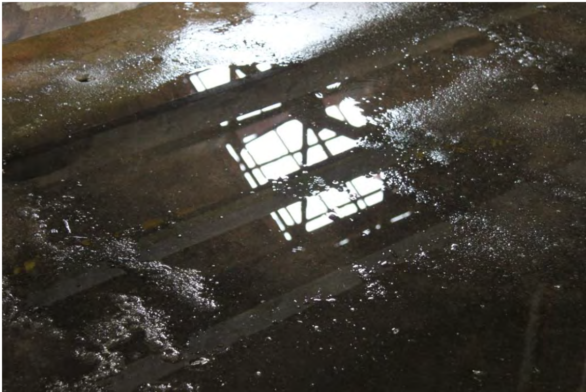
Figure A-11 Large roof openings have allowed water to leak through
