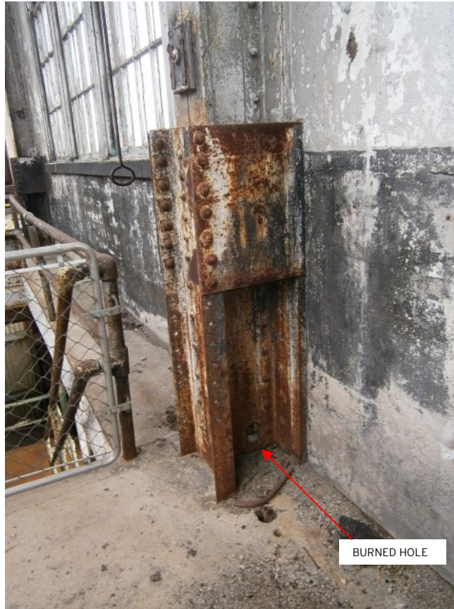
Photo #24: Burned hole through column web
