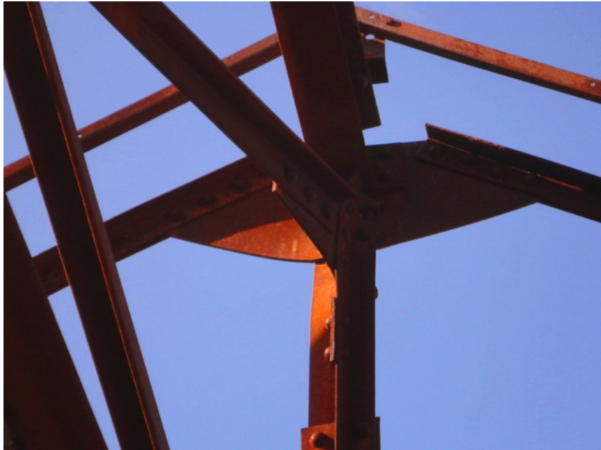
Photo #14: Typical steel corrosion in apex of roof in fire damaged region
