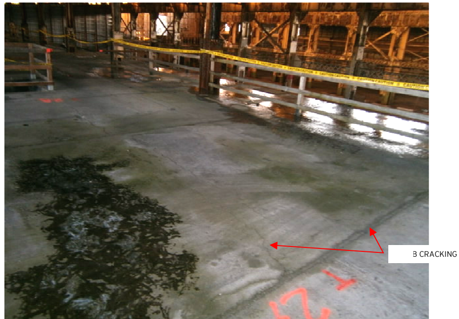
Photo #26: Typical mezzanine slab cracking
