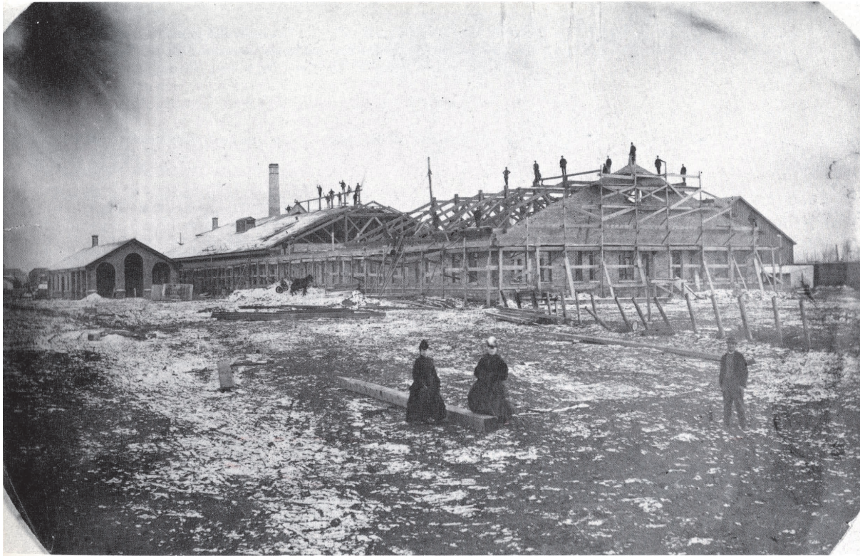
Above: The Grand Trunk Railway's new shop facilities under construction in the winter of 1870-71.
