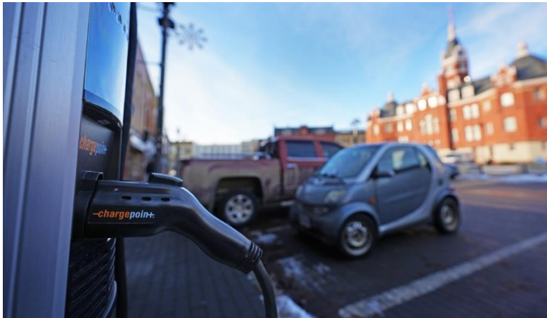
Figure 9 Electric vehicle (EV) charging station at Market Square
