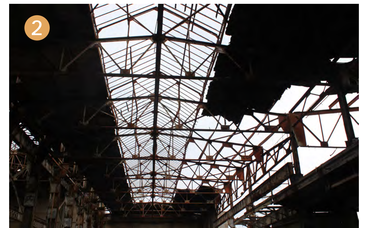
Cladding and roofing systems were found to be in poor to very poor condition.
