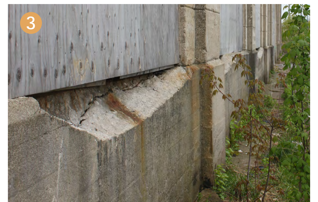
Severe deterioration, cracking and spalling concrete was observed.
