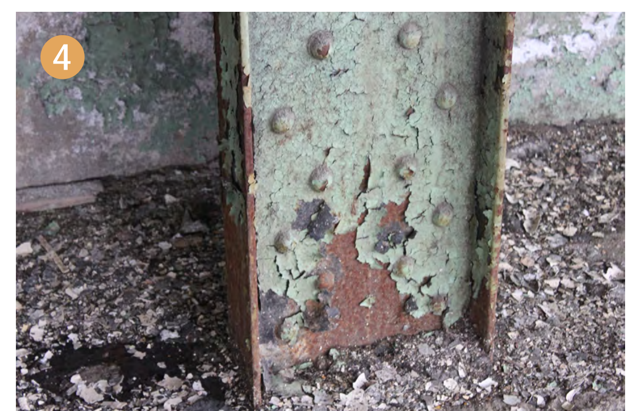
Corrosion is present at the base of columns.
