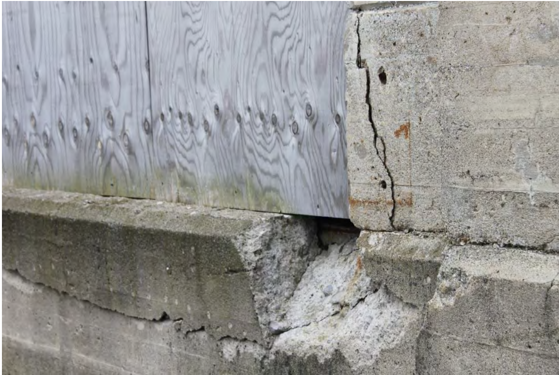
Figure A-14 View of deterioration and cracking
