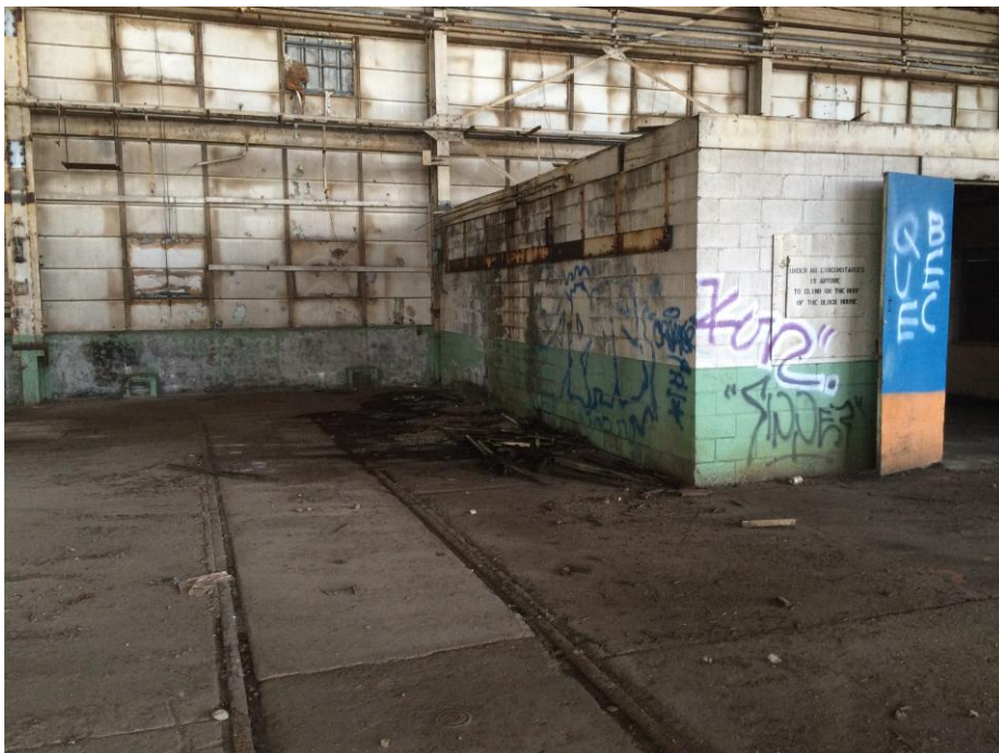
Photo #8: Roofing Debris Scattered Throughout the Site
