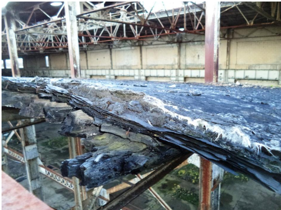
Photo #4: Typical Roof Deterioration
