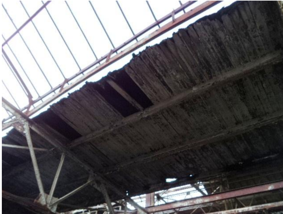
Photo #3: Typical Roof Deterioration
