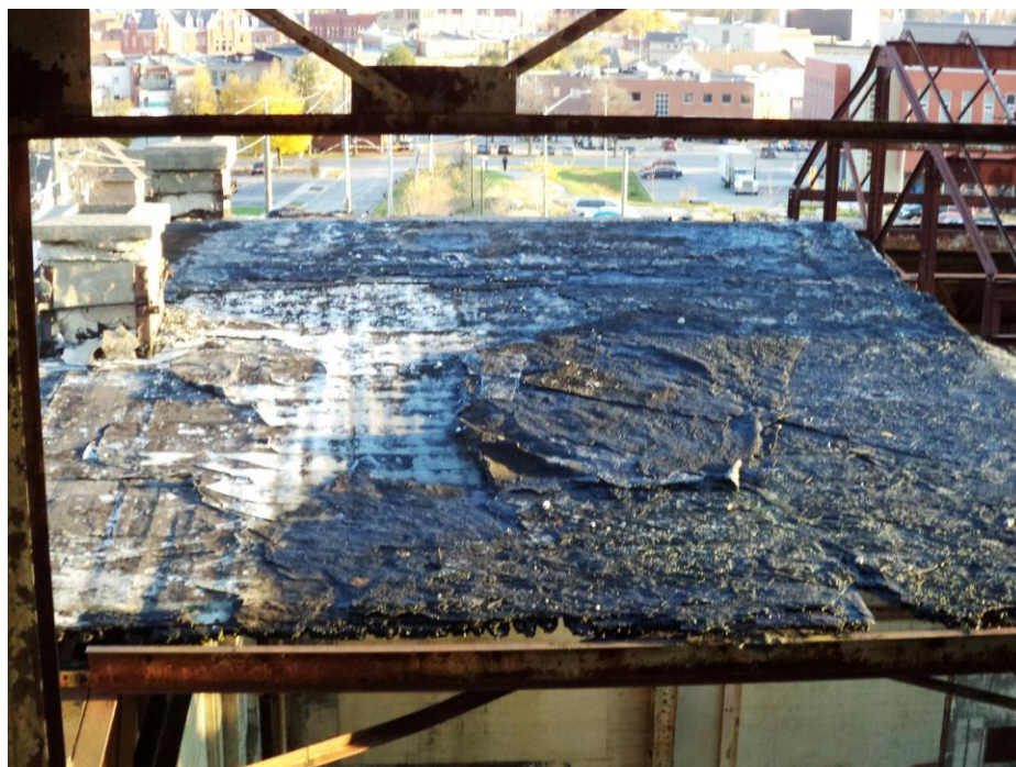
Photo #6: Typical Roof Deterioration
